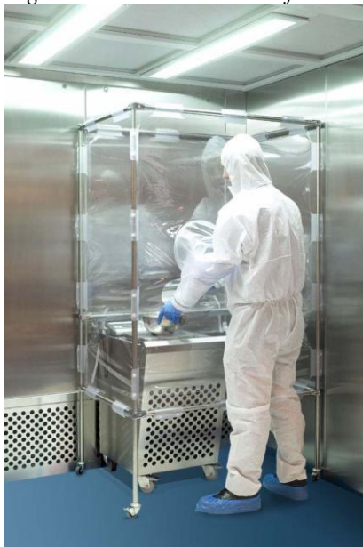
Figure 3.9.5 Partial screen fitted with glove ports inside a downward laminar flow booth
